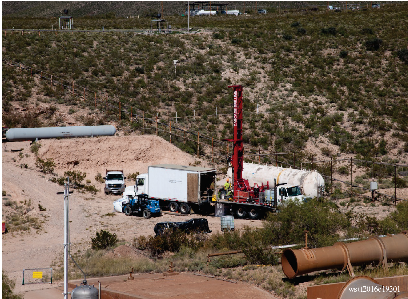
Set up for drilling on SB-15. The white support truck (facing left) is backed up to the drill rig, with the drilling platform supported between them. The core barrels are staged in the support truck. The drill rig has a rotating head which picks up the core barrels and screws them together.
