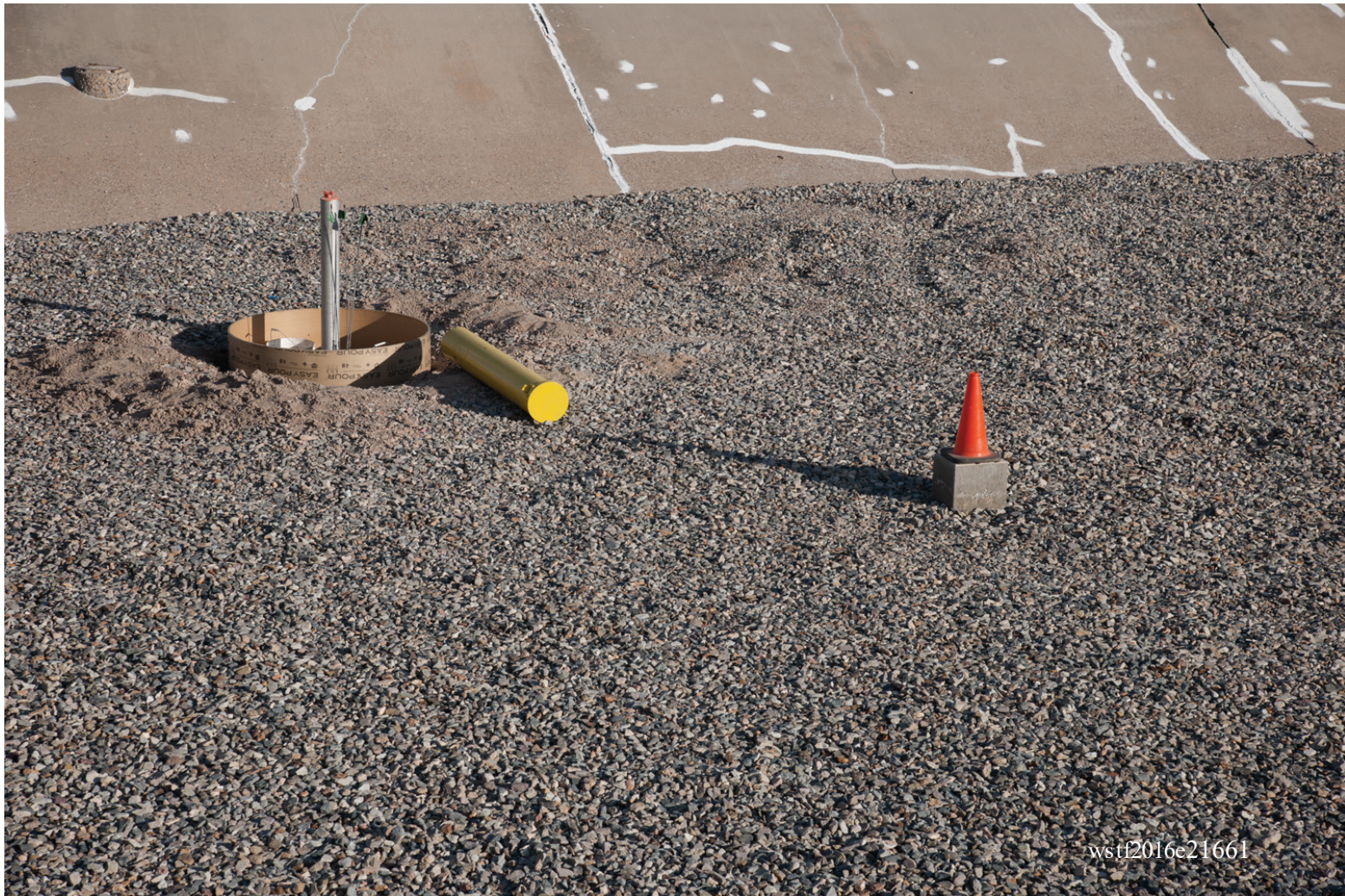
MSVGM well 400-EV-131 has been drilled, installed, and is ready for surface completion. The yellow steel protective stick up casing is lying to the right of the well. The 4 ft diameter cardboard tubing will be used to hold the concrete that will form the well pad.
