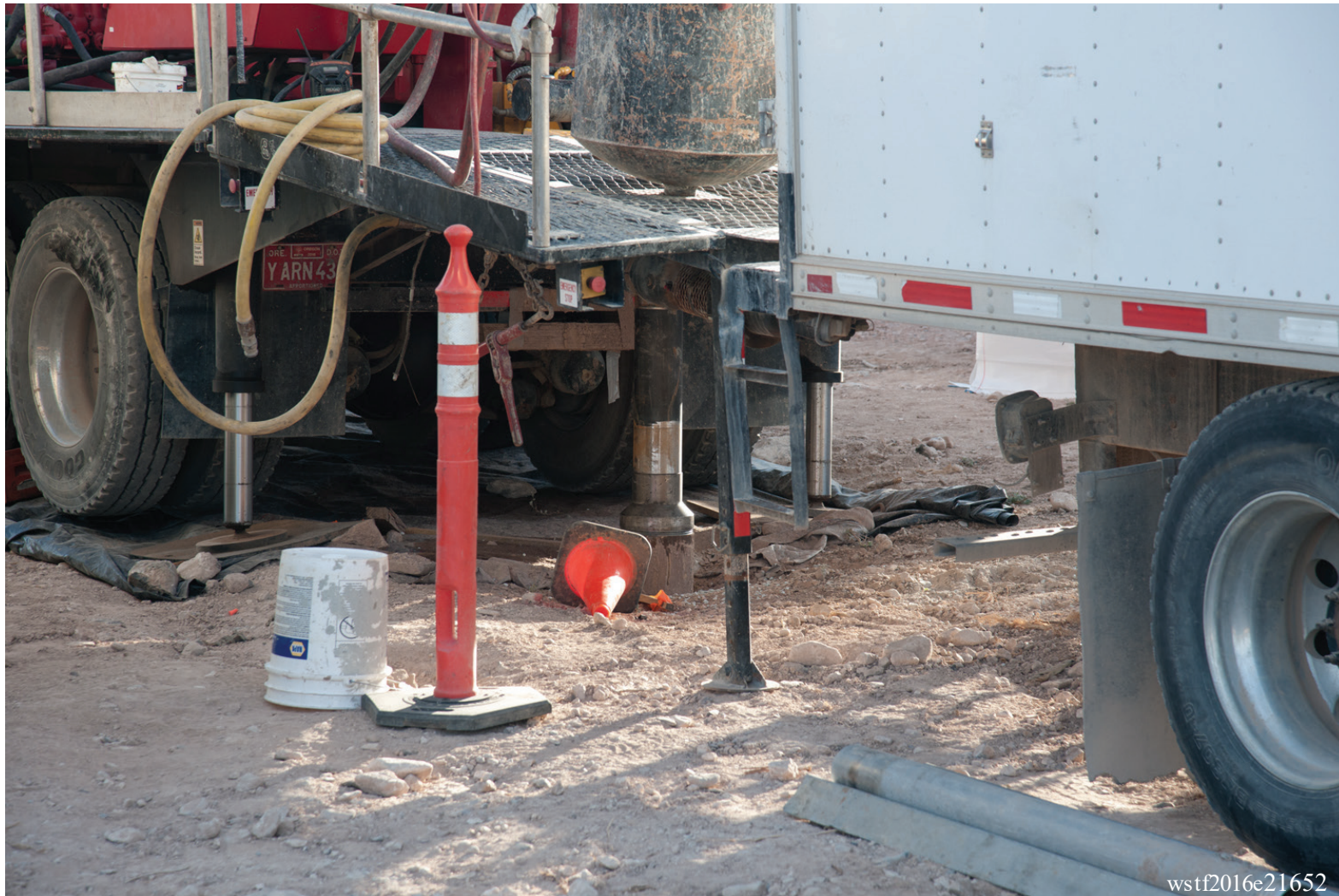
The drilling platform (steel grate) is set up between the drill rig and the support truck and supported by both. The top of a core barrel that has just been advanced can be seen above the surface.
