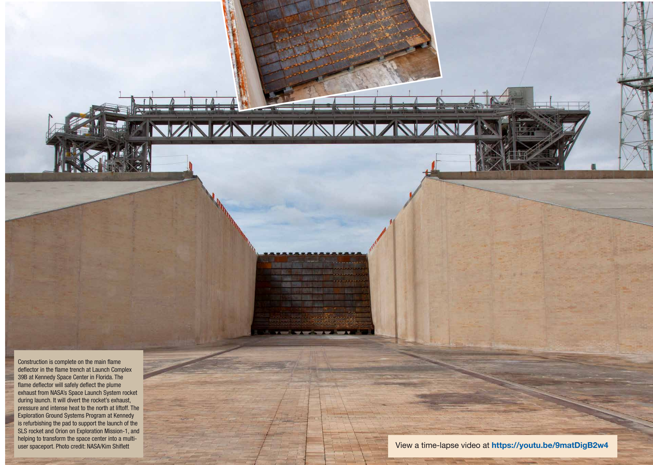
A close-up view of the main flame deflector in the flame trench at Launch Complex 39B at Kennedy Space Center in Florida. Photo credit: NASA/Kim Shiflett
