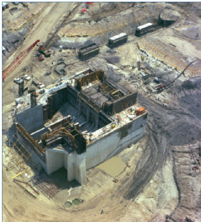
A 1960s photo shows construction of the Stennis A Test Complex, which tested rocket stages that helped land astronauts on the Moon in 1969.
