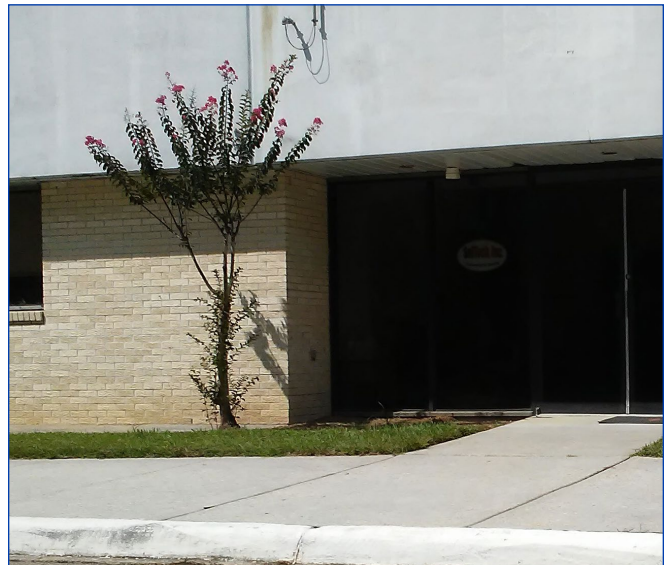
The sidewalk had been reported through the site's Close Call Reporting System as a safety fall hazard due to slipperiness.
