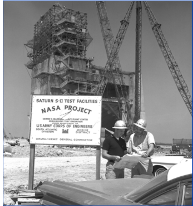
A 1965 construction site photo of the A-2 Test Stand at the Mississippi Test Operations site, known today as John C. Stennis Space Center.
