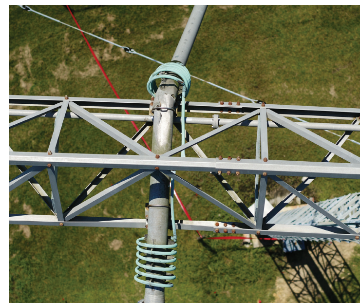
Stennis Space Center operators use drone images to safely inspect damage to an on-site high-frequency antenna Aug. 13, 2019, also reducing cost and saving time on repairs.
