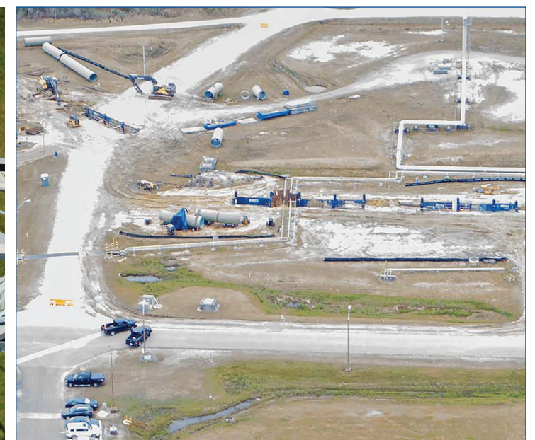
A drone captures high quality images Dec. 15, 2021, of an ongoing project to replace high-pressure industrial water lines in the A Test Complex at Stennis Space Center.
