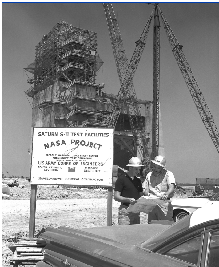
Construction of the A-2 Test Stand reaches higher and higher in early 1965 at Stennis Space Center, then-Mississippi Test Operations.
