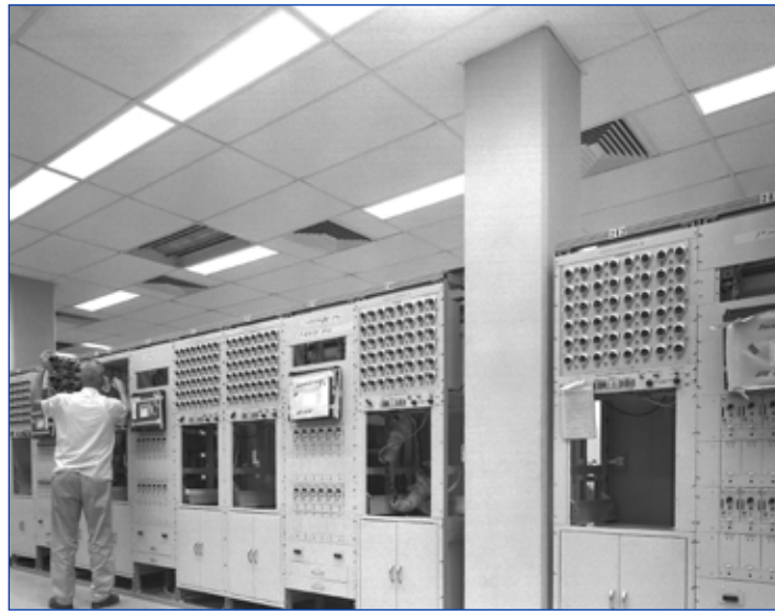
An employee works with Data Acquisition Facility instrumentation in 1965.
