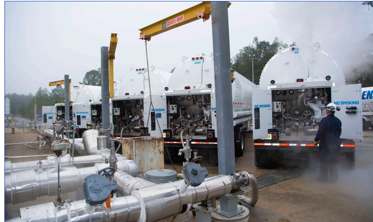
(Above photo) Tank trucks offload liquid gases at the Stennis high pressure gas facility during a test operations stress test Dec. 13.
