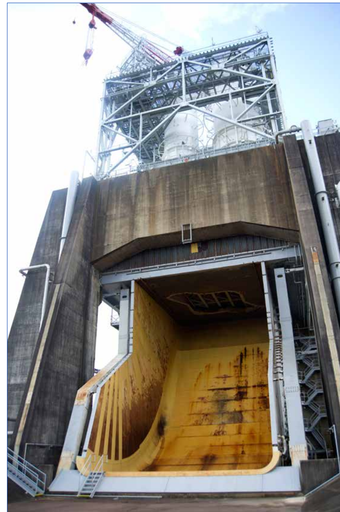
The A-1 Test Stand flame deflector, with the help of tens of thousands of gallons of pressurized water, plays a simple, yet important role in RS-25 rocket engine testing, directing ultra-hot exhaust safely out of the structure.
