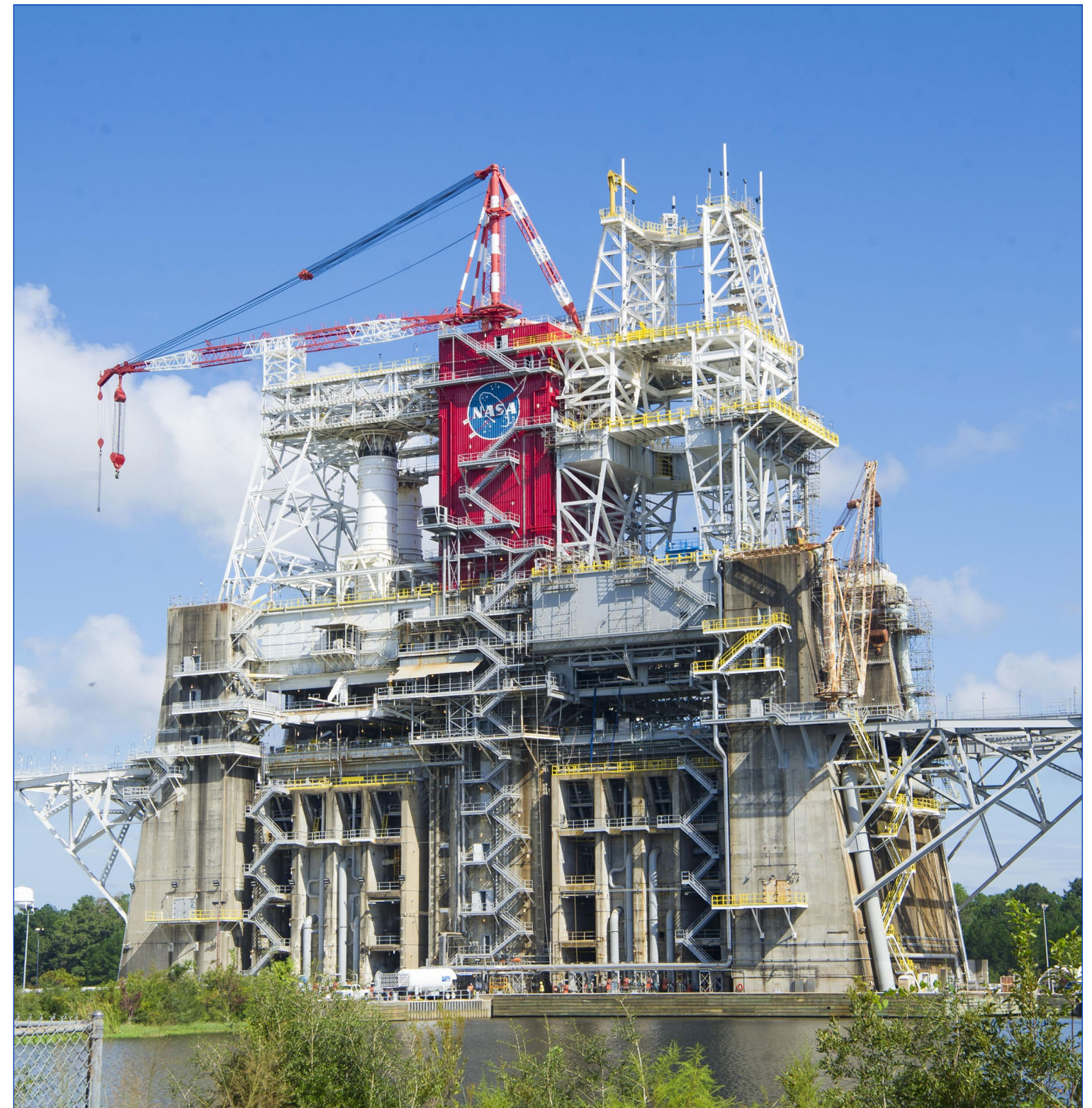
NASA plans to test the Space Launch System core stage that will help launch the Artemis 1 mission on the B-2 Test Stand at Stennis Space Center in 2020. Preparing for testing the SLS flight stage has required major modifications of all areas of the
