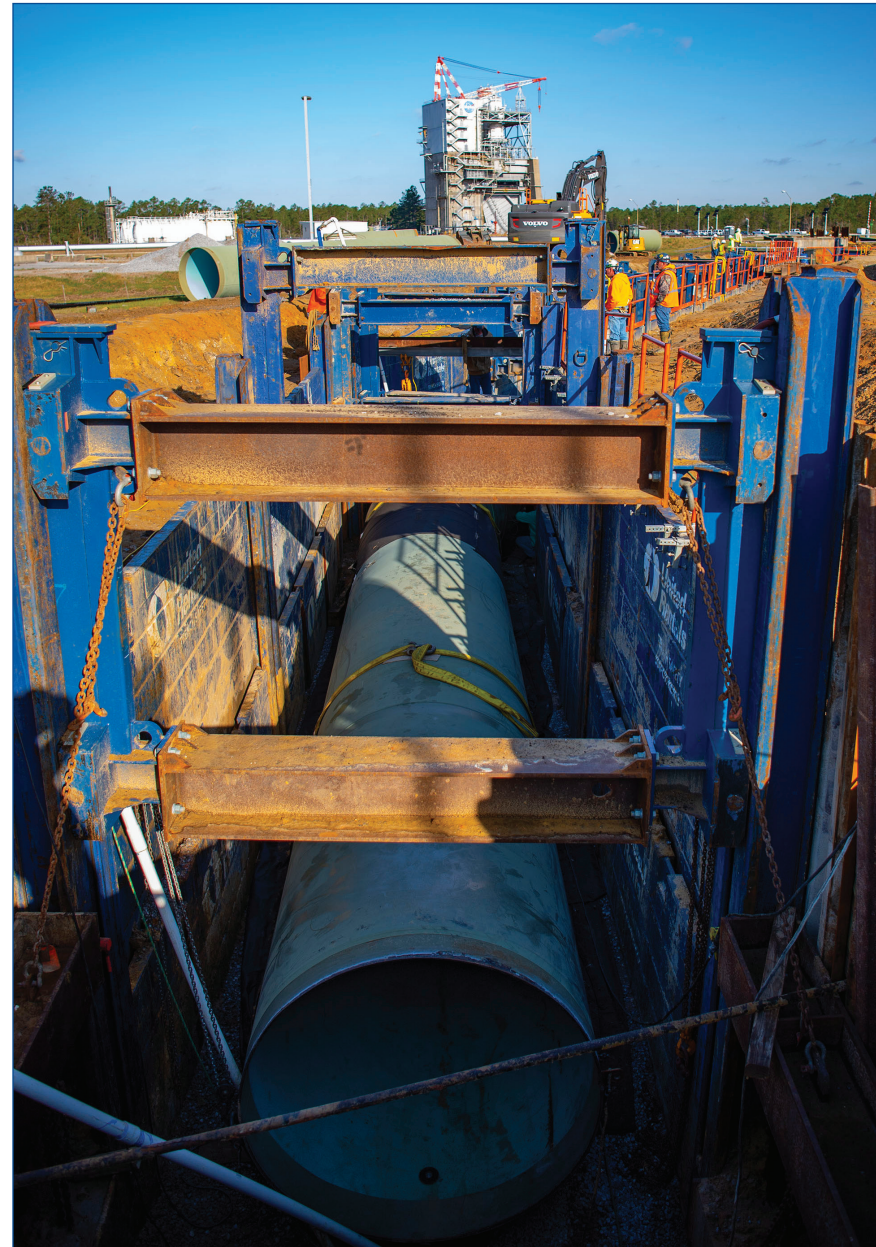
Crews use a shoring system to hold back soil March 23, 2022, as they install new 75-inch piping leading from the Stennis Space Center High Pressure Industrial Water Facility to the valve vault pit serving the Fred Haise Test Stand. The work is part of a critical infrastructure upgrade project.
