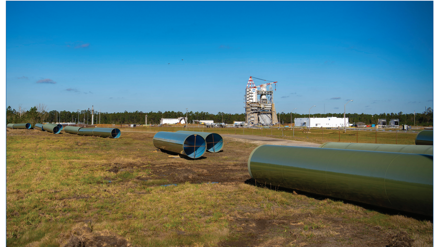
Sections of new 75-inch pipe await installation between Stennis Space Center's High Pressure Industrial Water Facility and the valve vault pit serving the Fred Haise Test Stand on March 23, 2022. Installation of the pipe is part of a critical upgrade for the center's aging infrastructure.
