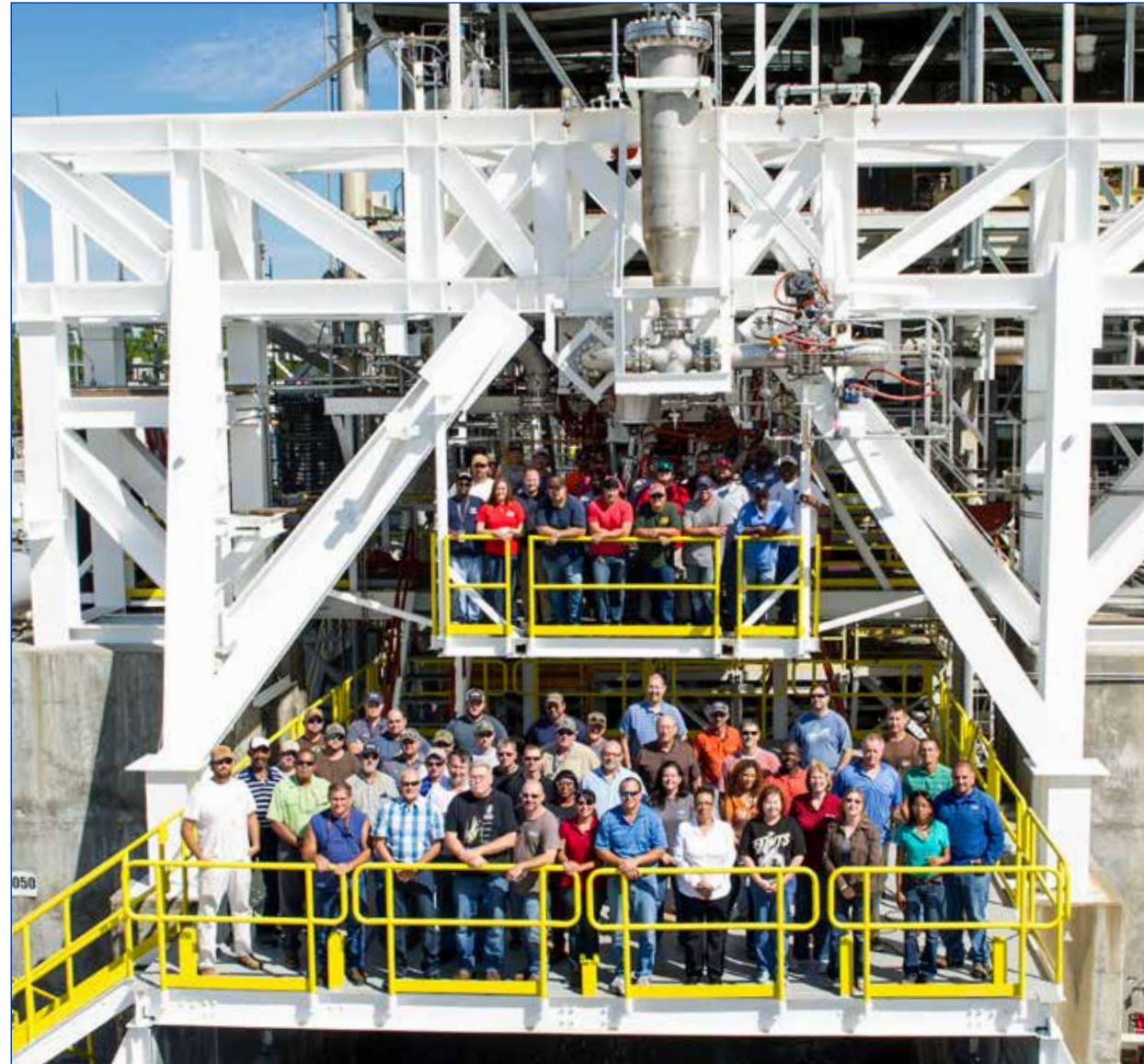
(Top photo) Members of work teams involved with repair of the E-1 Test Stand following damage from a May fire stand at the facility. Thanks to team efforts, repair work on the stand was completed weeks earlier than initially estimated.
