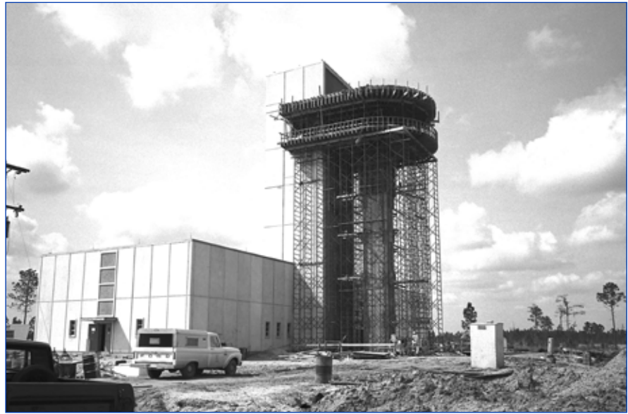
Progress proceeds in March 1965 on construction of Building 1200 at Stennis Space Center, once known as the Central Control Building.
