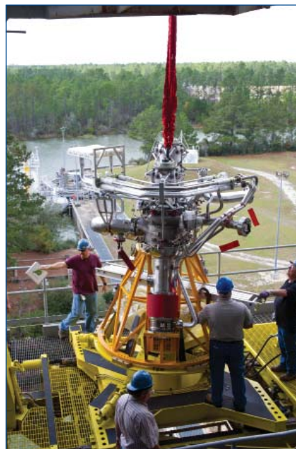
Stennis employees prepare to install the J-2X powerpack on the A-1 Test Stand.
