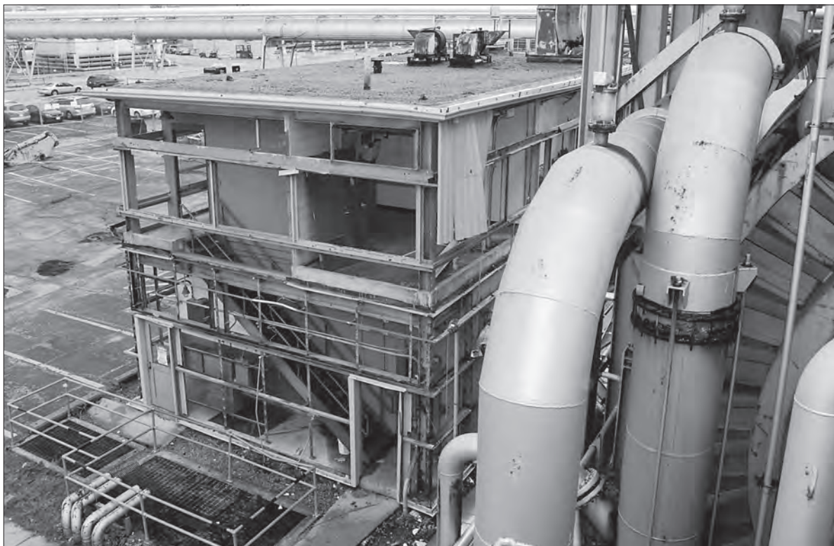
Image 158: The Service Support Building's exterior walls are removed in September 2008 as one of the first steps in the demolition of PSL No. 1 and 2. (NASA C-2008-04132)
