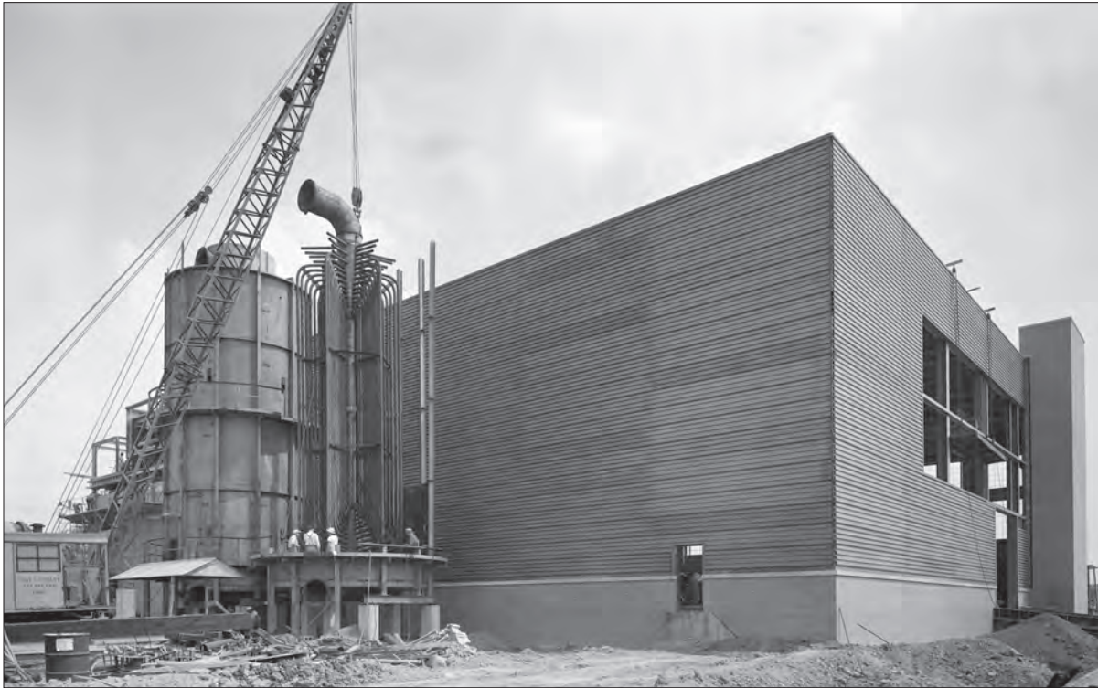
Image 31: Construction of the gas-fired air heaters outside the Equipment Building on 29 August 1951. (NASA C-2009-00163)
