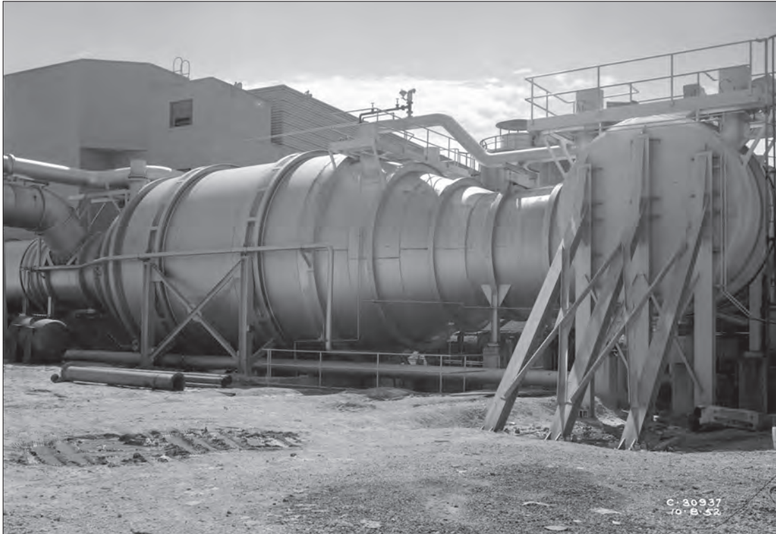
Image 68: The airflow was then pumped through a secondary cooler, seen here on 8 October 1952. This secondary cooler cooled and scrubbed the exhaust gases from both test chambers to reduce explosion hazards before the gases were pumped through the exhausters in the Equipment Building and expelled into the atmosphere. 17 (NASA C-1952-30937)
