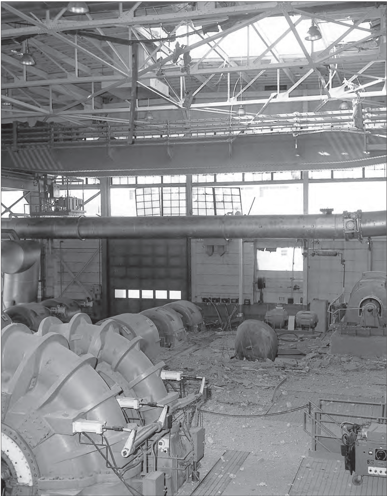
Image 127: Overall interior view on 7 April 1971 of damage from the PSL Equipment Building explosion. Note the broken windows in the far wall, the hole in the roof, and the raised heater at the floor level surrounded by debris. (NASA C-1971-01272)
