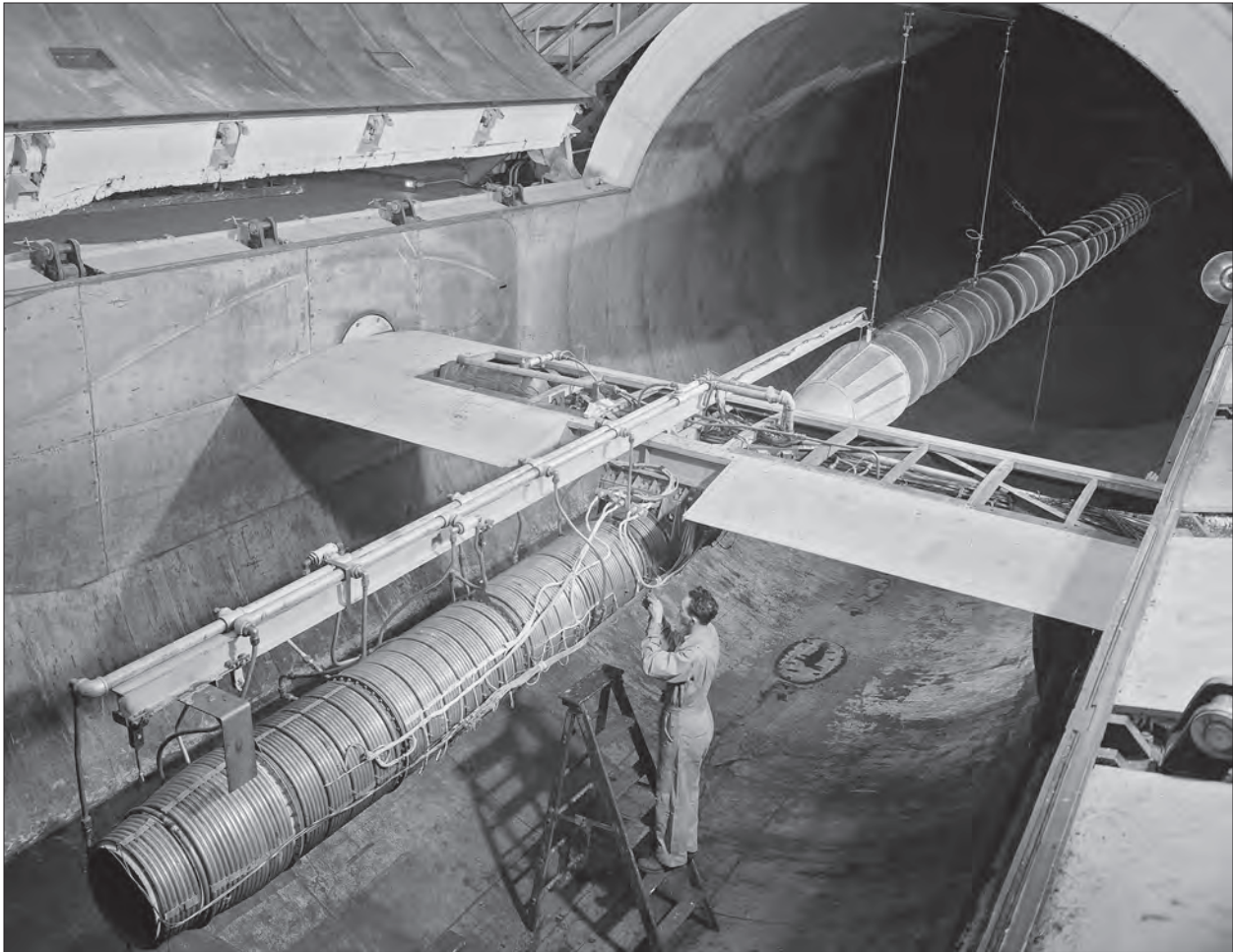
Image 10: An NACA-designed ramjet engine with afterburner is installed in the AWT on 7 February 1946. To produce the proper settings, researchers changed the design so that the conditioned air was ducted directly to the engine's inlet. (NASA C-1946-14244)
