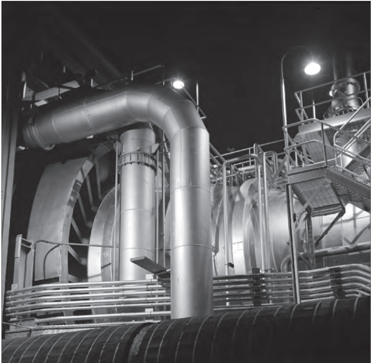
Image 36: PSL No. 1's primary cooler as it appeared on 24 September 1952, just after completion. After months of calibration, the PSL was about to commence testing. (NASA C-1952-30767)
