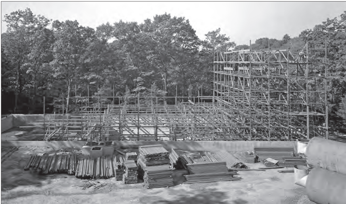
Image 32: Construction of the wooden PSL Cooling Tower in a wooded area across the road from the PSL in September 1949. (NASA C-2009-00161)
