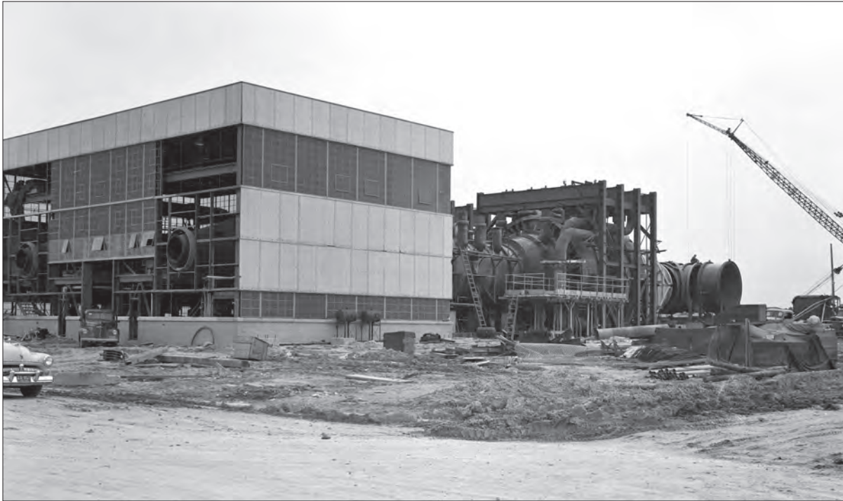
Image 28: The Shop and Access Building during construction in May 1951. The two portals on the front would later permit conditioned air to be piped into the two altitude chambers inside. (NASA C-2009-00195)
