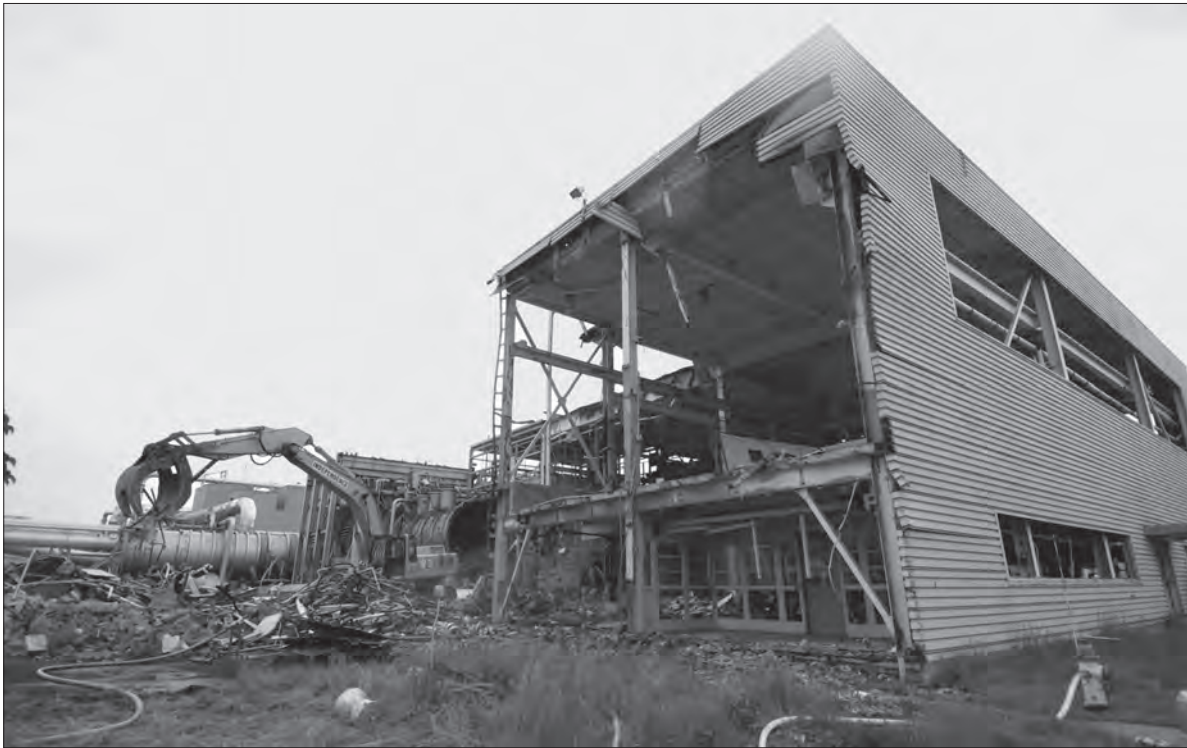
Image 159: A steam shovel tears apart the PSL Shop and Access Building on 3 June 2009. (NASA C-2009-01660)
