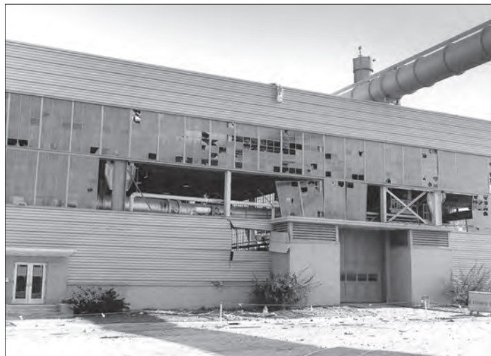
Image 126: An overpressurization in the exhausters in PSL's Equipment Building caused a serious explosion. This 7 April 1971 photograph shows windows blown out on the exterior of the building. (NASA C-1971-01269)
