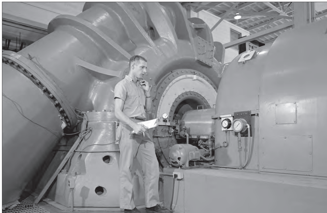
Image 65: An equipment operator examines an exhauster on 15 August 1963. The original configuration could remove the gases at a rate of 100 pounds per second when the simulated altitude was 50,000 feet. Each of the thirteen 5,100-horsepower exhauster units contained two J33 compressor wheels that could be adapted to work in tandem or parallel. The number of units used could be varied to control the power load. 16 (NASA C-1963-65822)
