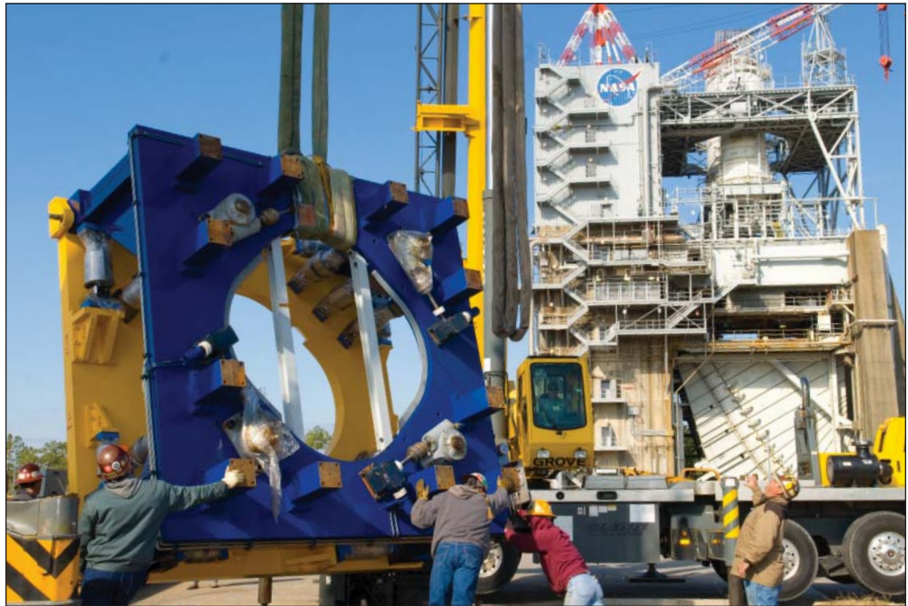
(Top photo) Stennis Space Center employees maneuver a new thrust measurement system in preparation for its installation on the A-1 Test Stand on March 3. The system was fabricated by Thrust Measurement Systems in Illinois and represents a state-of-the-art upgrade from the equipment used on the stand for more than 40 years.
