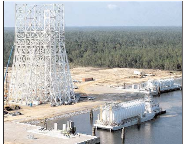
A fuel barge pulls up to a new A-3 Test Stand transfer dock during a July 9 test of the structure's pin anchoring system.
