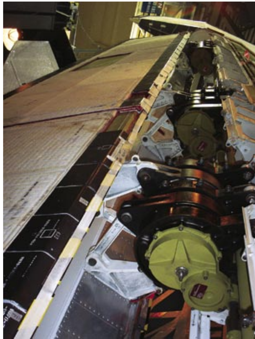
Looking up at an Orbiter's vertical stabilizer. Three rudder/speed brake actuators are visible.
