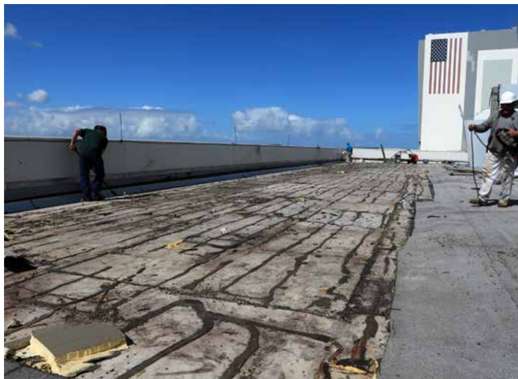
(Below) Members of the Disaster Assessment and Recovery Team (DART) repair a section of roof atop Kennedy's Operations Support Building II, part of the spaceport's recovery from Hurricane Matthew.
