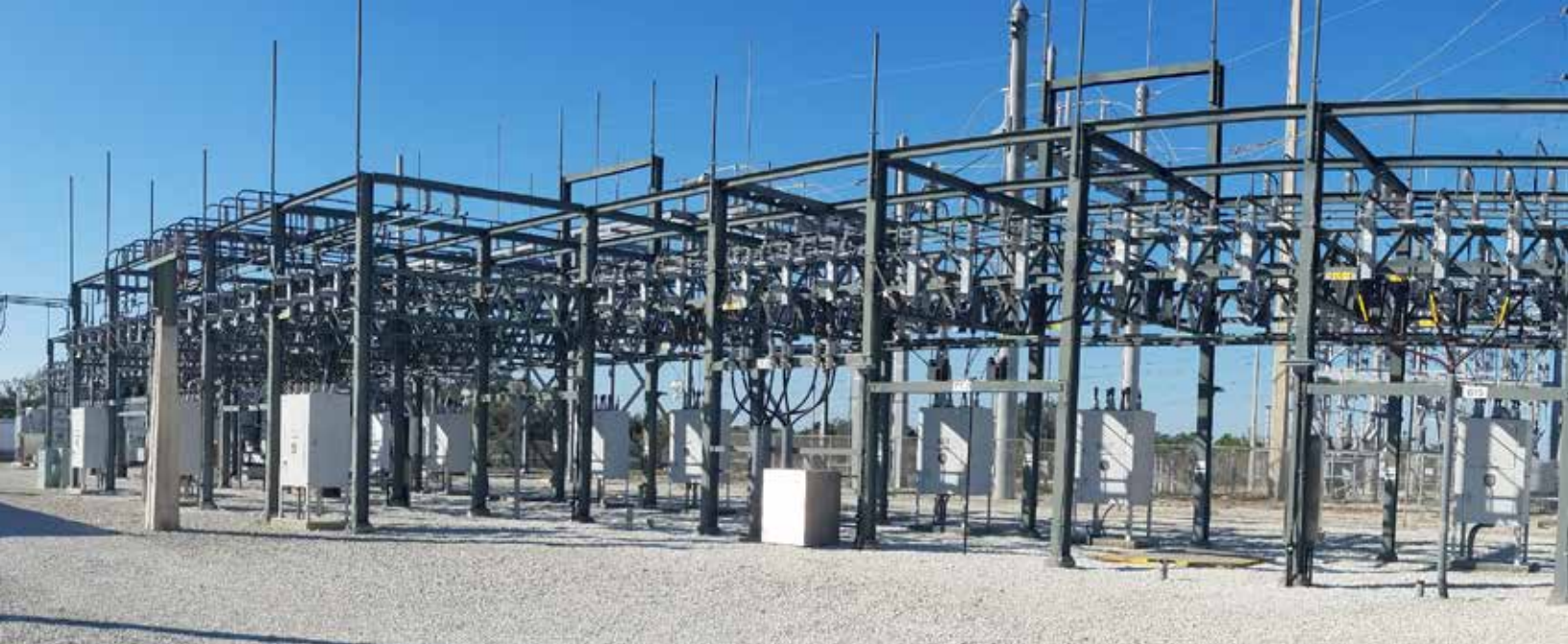
(Above) Kennedy Space Center's C5 power substation is seen in this wide-angle photo. The spaceport's electrical power infrastructure is being revitalized and upgraded.
