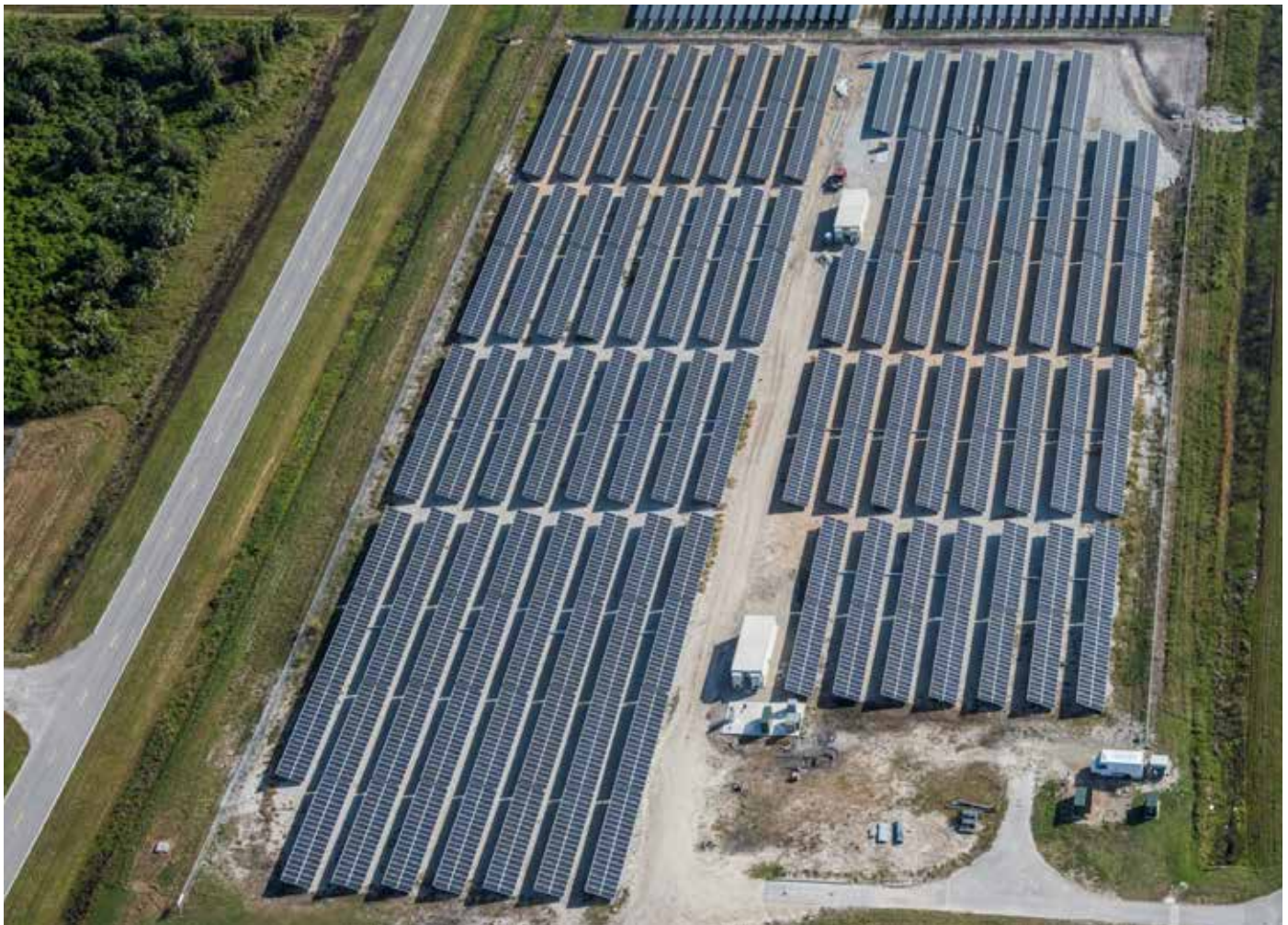
Construction of a second solar plant is nearing completion. This addition will enable the center's new Headquarters building to achieve net-zero energy consumption while also satisfying Kennedy's commitment to meeting the agency's renewable energy goals.
