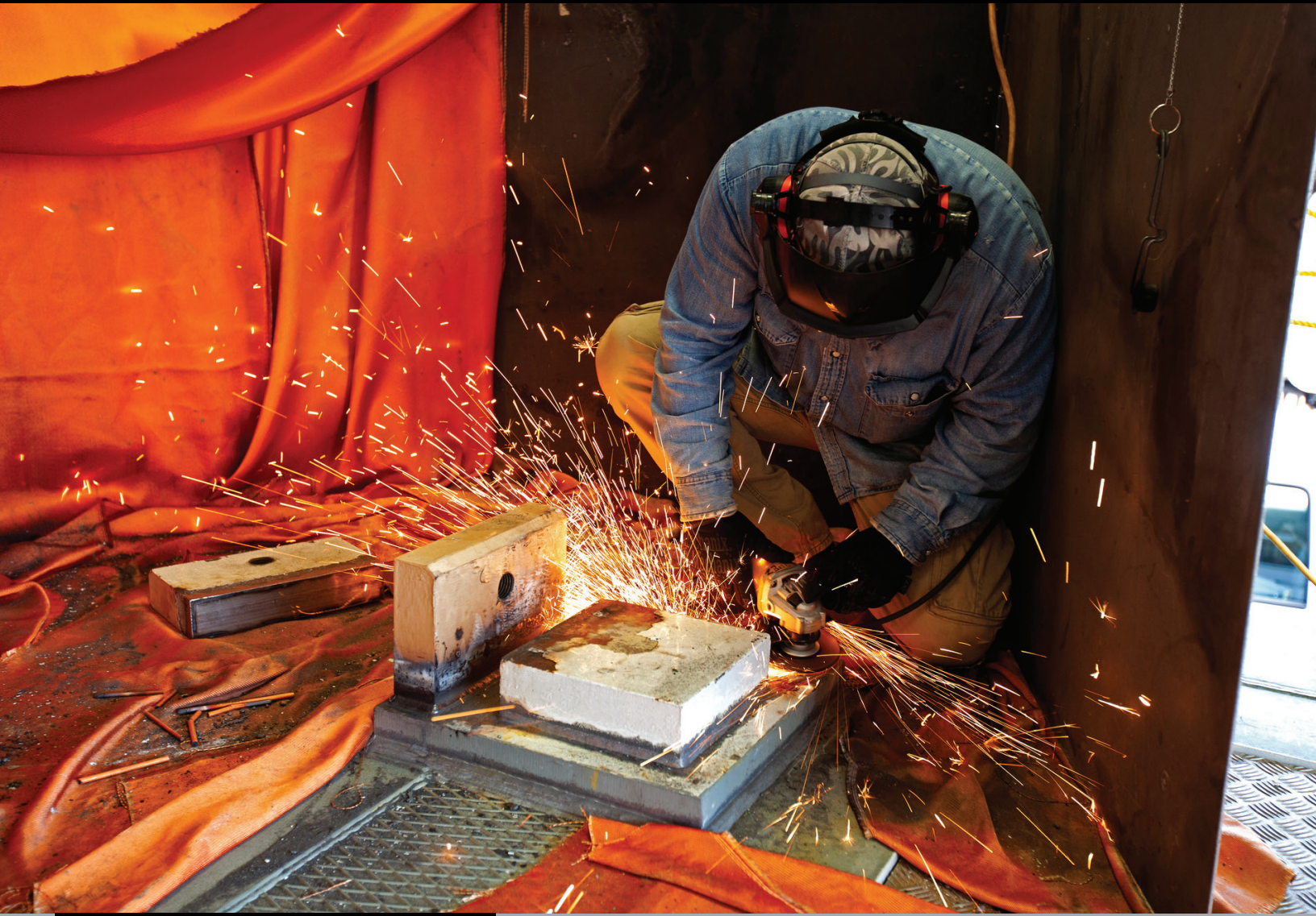
A Jacobs technician from the Launch Equipment Shop performs welding on the KAMAG spacecraft transporter on Oct. 26, 2018, inside a facility at the crawler yard at NASA's Kennedy Space Center in Florida. The transporter is designed to carry heavy loads. Welding is being performed on the attach points that will hold the Orion transportation pallet in place. Testing of the pallet will be performed to support validation and verification of the attach fittings in the Multi-Payload Processing Facility. Photo credit: NASA/Ben Smegelsky
