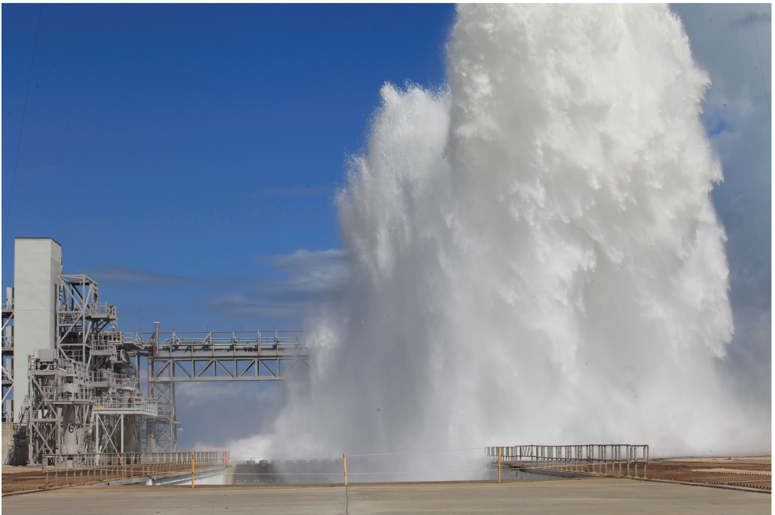
A flow test of the Ignition Overpressure Protection and Sound Suppression water deluge system was completed at Launch Pad 39B on Oct. 15, 2018, at NASA's Kennedy Space Center in Florida.
