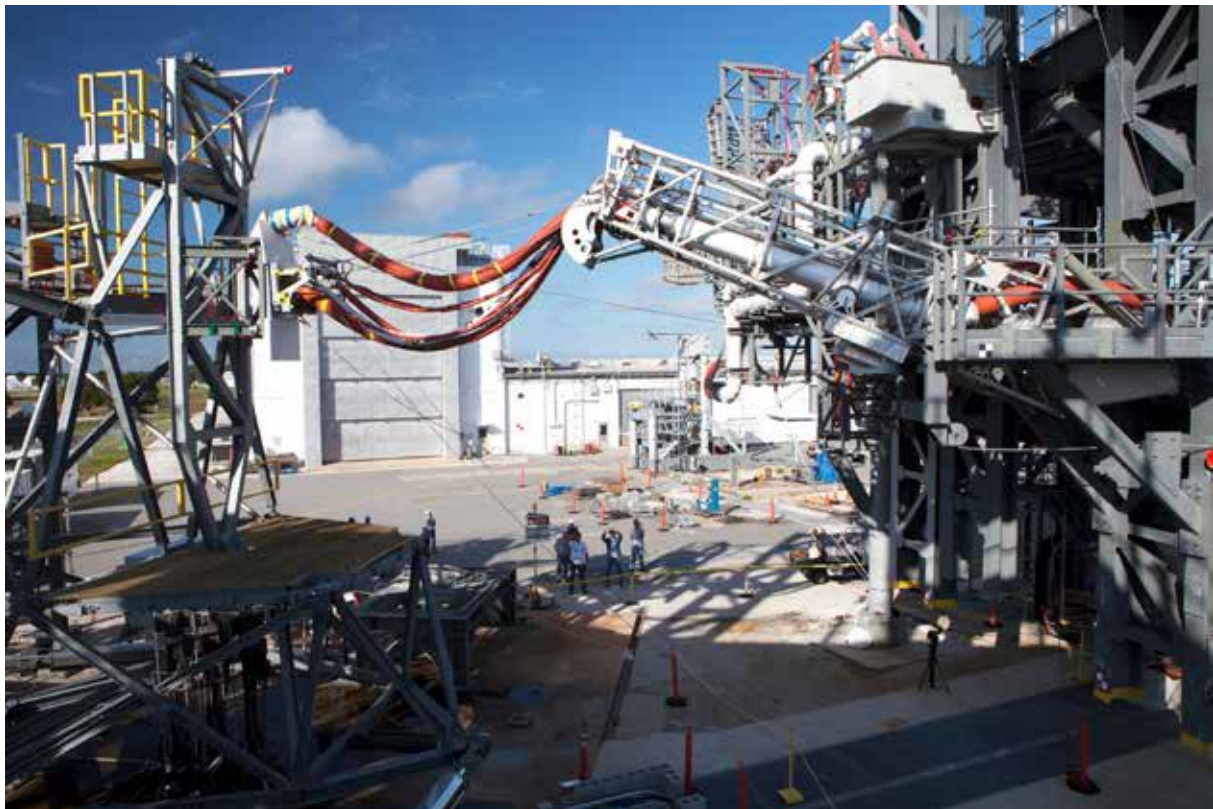
The Orion Service Module Umbilical (OSMU) lines were connected to Vehicle Motion Simulator 1 on Dec. 16, 2015, to begin a series of tests, including a simulated launch test, at the Launch Equipment Test Facility at Kennedy Space Center. The center's Engineering Directorate is providing support to the Ground Systems Development and Operations Program for testing of the OSMU and other umbilical lines.
