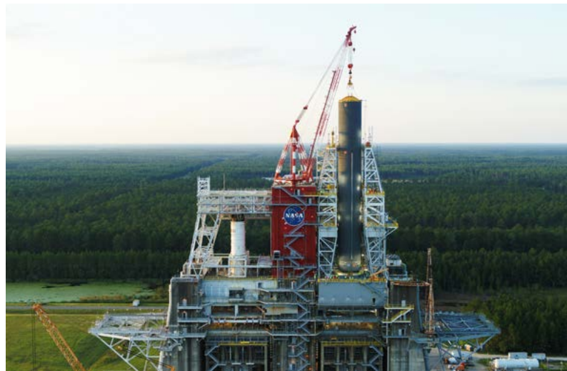
NASA’s Space Launch System core stage pathfinder is positioned in the B-2 Test Stand at Stennis Space Center on September 27, 2019, in preparation for the Green Run test series. Photo credit: NASA
