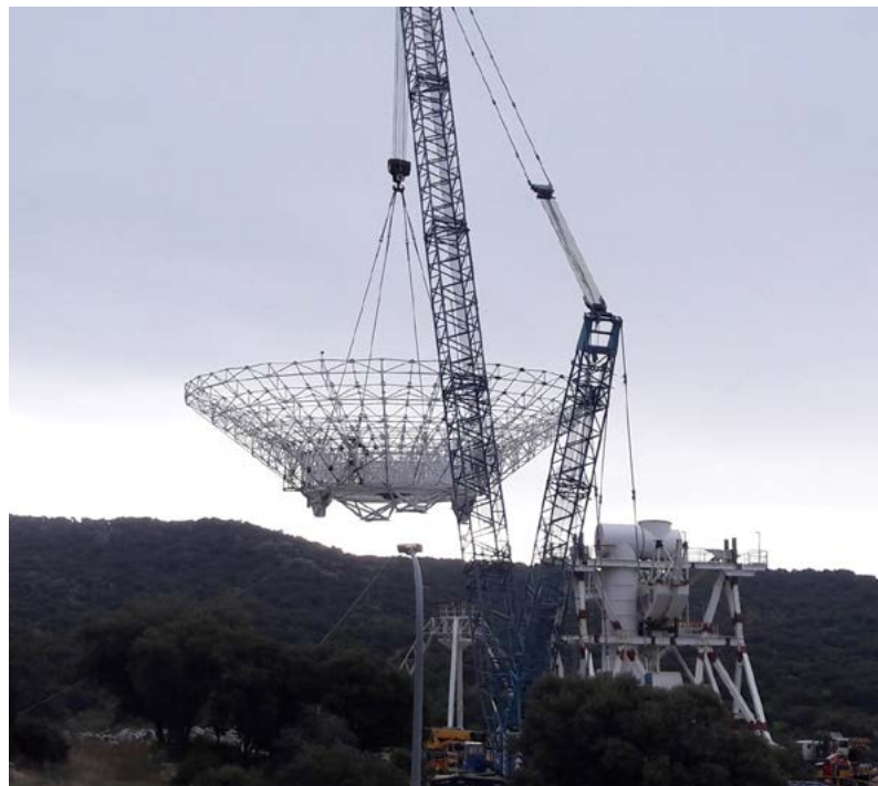
The antenna reflector for DSS-56 is hoisted onto its pedestal in November 2018. DSS-56 is one of the newest 34-meter antennas under construction at MDSCC. Photo credit: NASA/Centro de Entrenamiento y Visitantes
