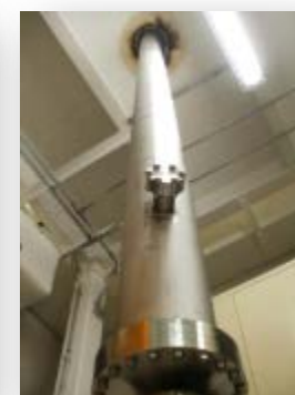
Cryogenic Container located at MSFC (below deck)
