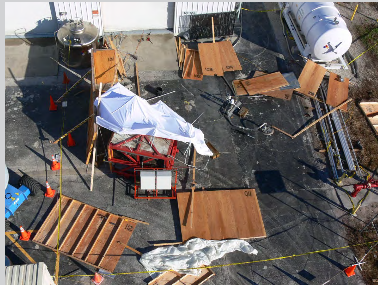
The aftermath of the composite pressure vessel that burst during cryo testing at Kennedy Space Center's Cryogenics Laboratory On Dec. 23, 2008. Photo credit: NASA
