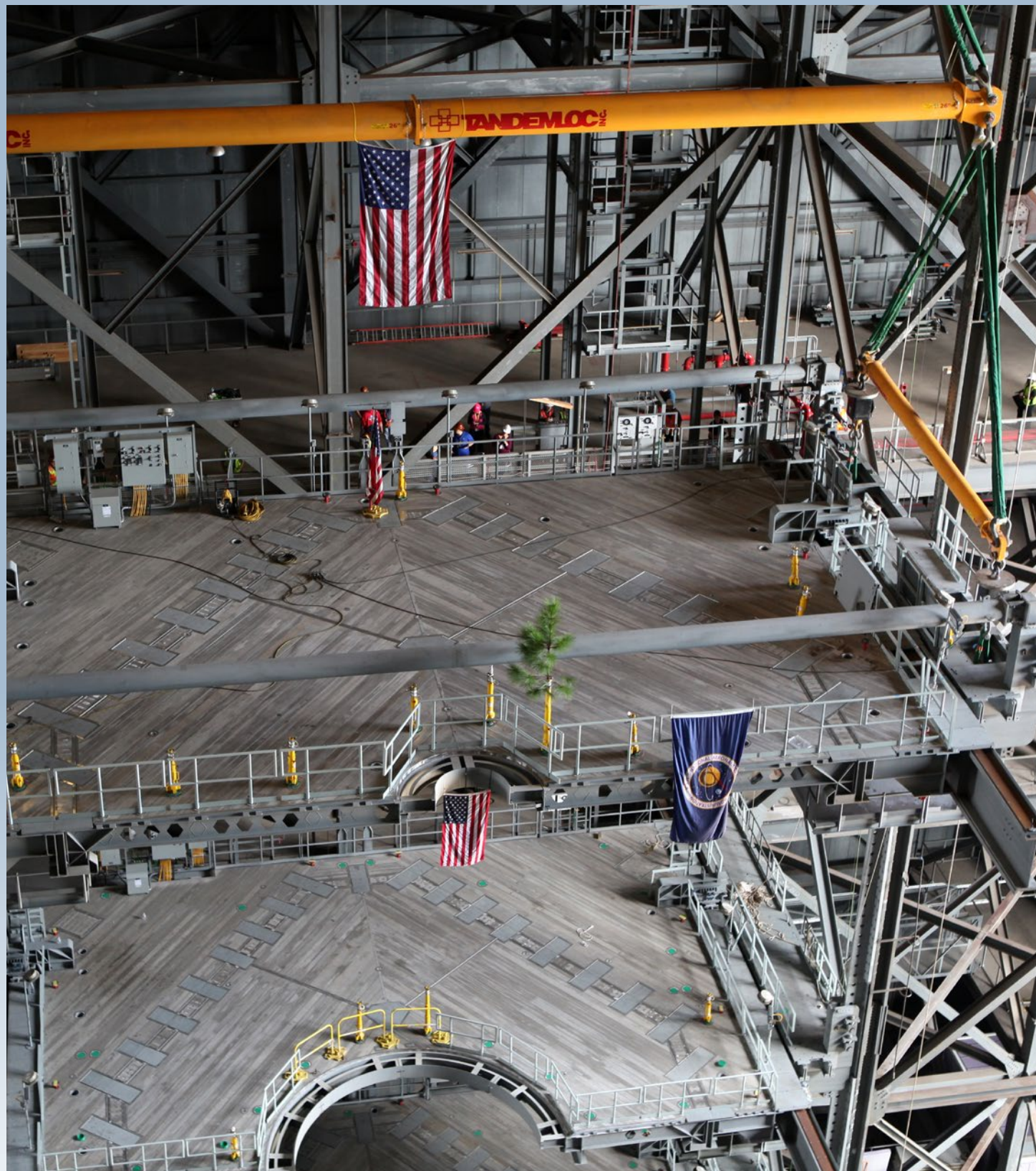
High up in the Vehicle Assembly Building (VAB) at Kennedy Space Center, a crane lowers the final work platform, A north, for installation in High Bay 3. The platform was installed and secured on its rail beam high up on the north wall of the high bay. In view on the platform are the American flag and a small tree. The installation of the final topmost level completes the 10 levels of work platforms, 20 platform halves altogether, that will surround NASA's Space Launch System rocket and the Orion spacecraft and allow access during processing for missions, including the first uncrewed flight test of Orion atop the SLS rocket in 2018. Photo credit: NASA/Frank Michaux
