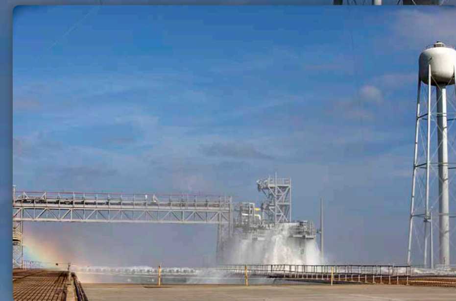
Water flowed at high speed from a holding tank through piping and valves, the flame trench and mobile launcher interface risers during a wet flow test at Launch Pad 39B at NASA's Kennedy Space Center. Photo credit: NASA/Kim Shiflett
