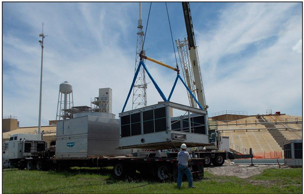
One of two new 400-ton-plus capacity cooling towers arrives at Launch Pad 39B at NASA's Kennedy Space Center Florida in July 2014. The two cooling towers will feed three new 180-ton-capacity chillers for the heating, venting and air conditioning system. Photo credit: NASA
