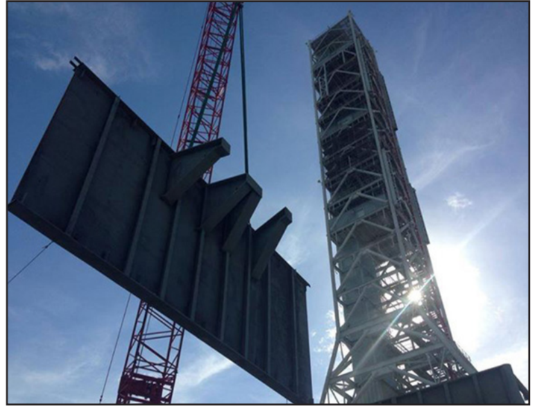
A crane is used to lift one of the heavy steel girders for installation on the mobile launcher at the Mobile Launcher Park Site. Photo credit: JP Donovan
