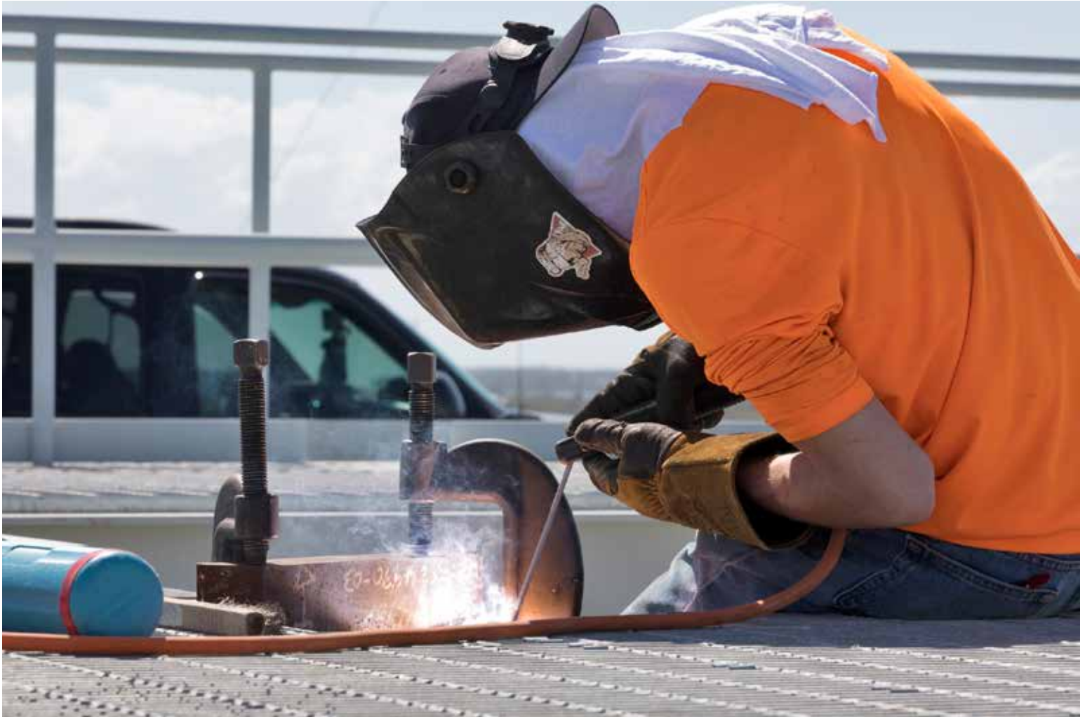
A construction worker welds a section of metal on the surface of Launch Pad 39B at NASA's Kennedy Space Center in Florida on February 22, 2019.
