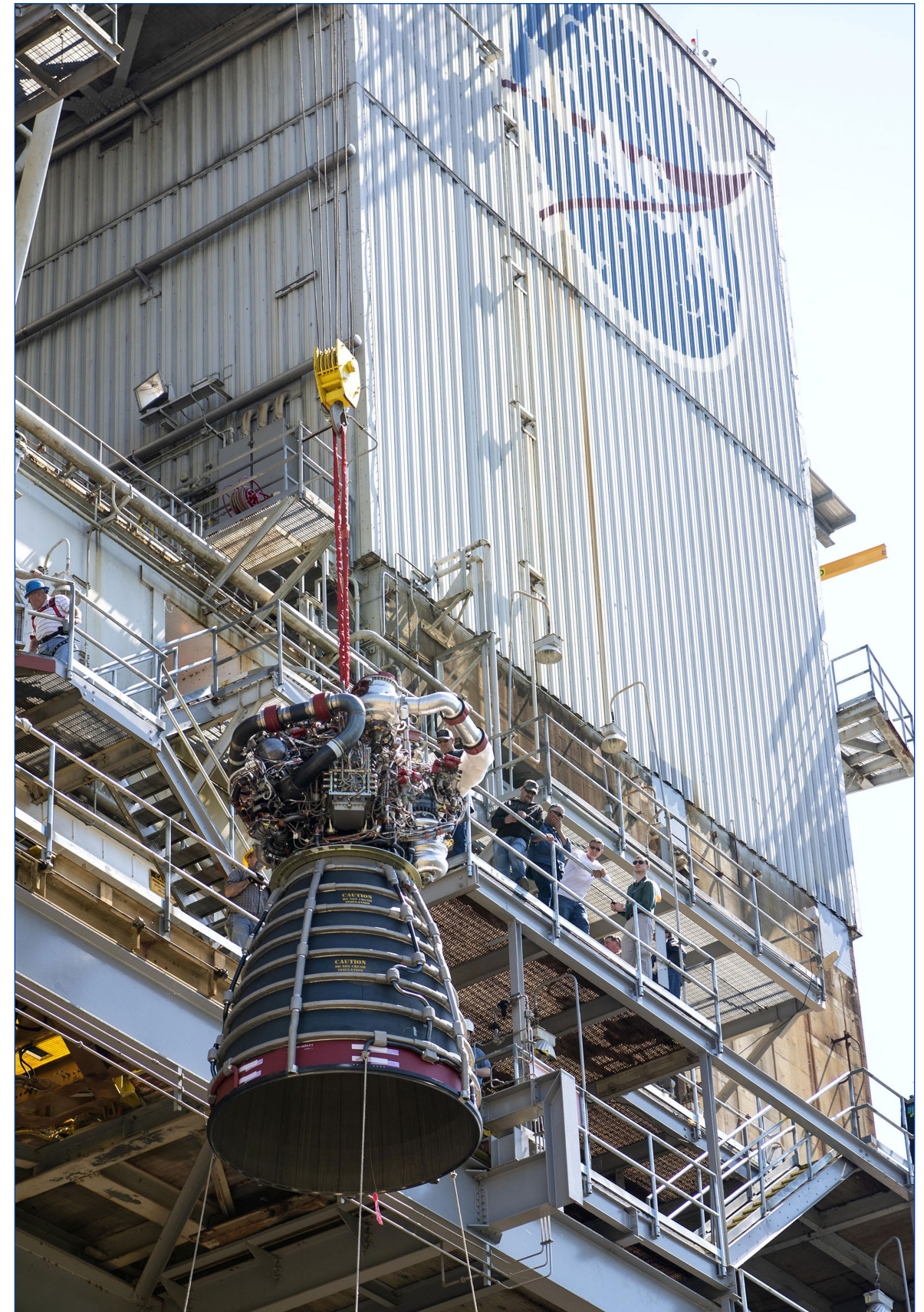
RS-25 flight engine No. 2062 is lifted onto the A-1 Test Stand at NASA's Stennis Space Center near Bay St. Louis, Miss. The Aerojet Rocketdyne-built engine was delivered to the stand March 20 and test fired April 4.
