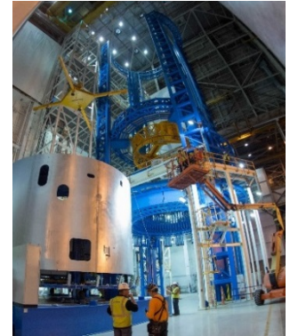
Vertical Assembly Center
