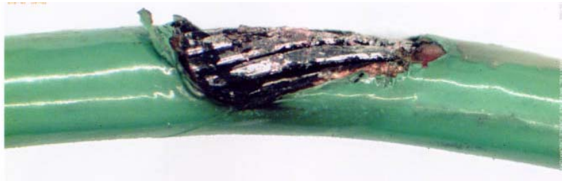
Figure 2: Damaged wire that resulted from a short to ground on the space shuttle.
