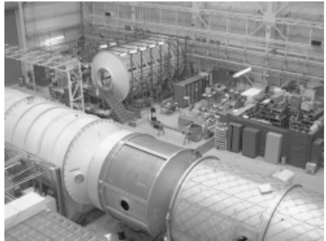
MSFC ECLSS Test Facility
