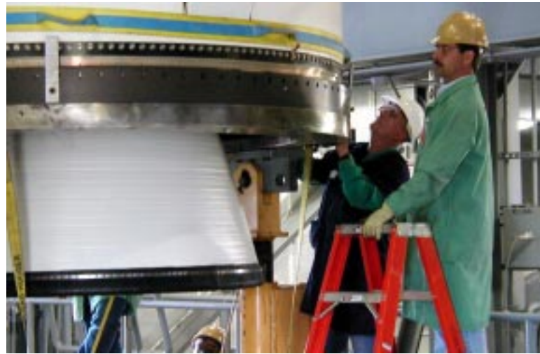
Technicians work on the Athena I rocket that will launch the Kodiak Star payload from Kodiak, Alaska.
