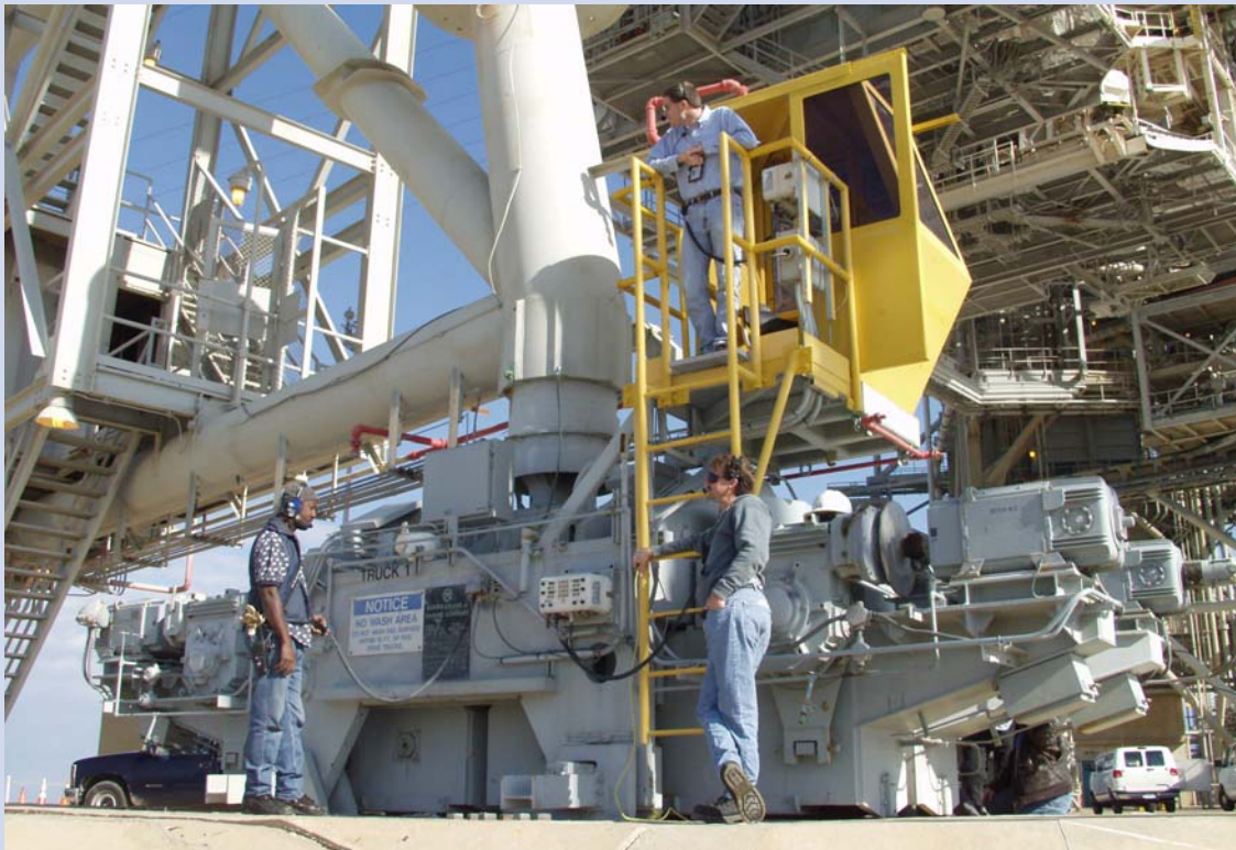
Alonzo Guinyard, Nathan McGowan and Ed Griffin of United Space Alliance help support an upcouple test of the Rotating Service Structure at Pad B.
