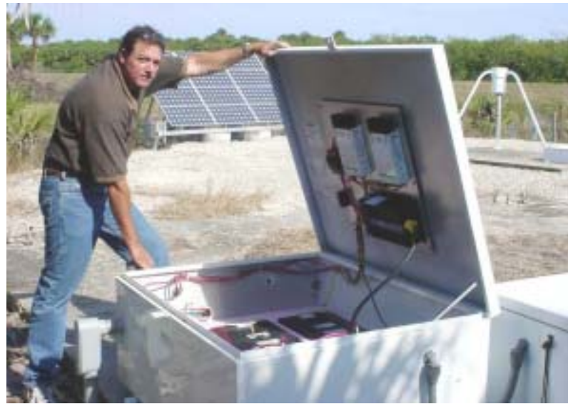
JOHN BROUGHTON (left) of Space Gateway Support's Energy Management Office explains how the Launch Pad Lightning Warning System (LPLWS) is powered. The LPLWS gives forecasters information on trends in electric field potential and the locations of highly charged clouds capable of supporting lightning. Below, SGS mechanical engineer Kevin Riley explains how the system is crucial because it protects all aspects of launches, including the vehicle, from potentially damaging lightning strikes.
