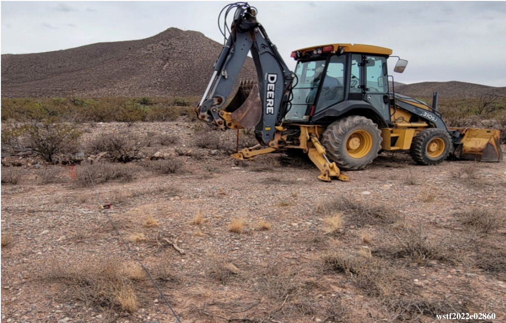
Northeast end of enhanced passive seismic survey line adjacent to 700 Area Landfill cap fence with backhoe energy source (view to the northeast [May 25-27, 2021]).
