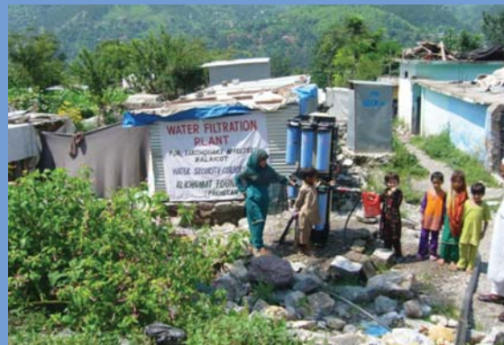
Water filtration plant in Balakot, Pakistan, that was set up following the earthquake disaster in 2005. The unit processes water using gravity fed from a mountain stream.
